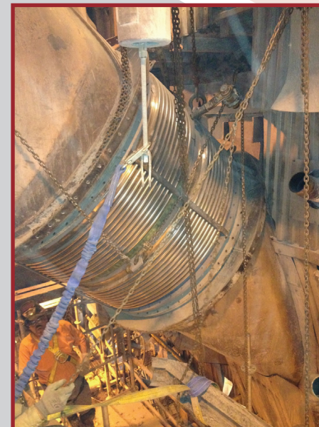
INCONEL 625 1800°F REFRACTORY LINED
