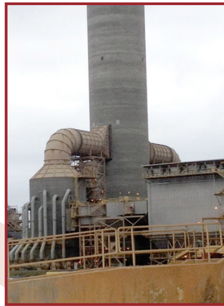
EXPANSION JOINTS SCRUBBER OUTLET TO THE STACK
