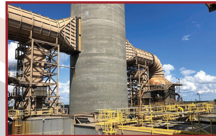
TWO SCRUBBER UNITS WITH EXPANSION JOINT SCRUBBER
